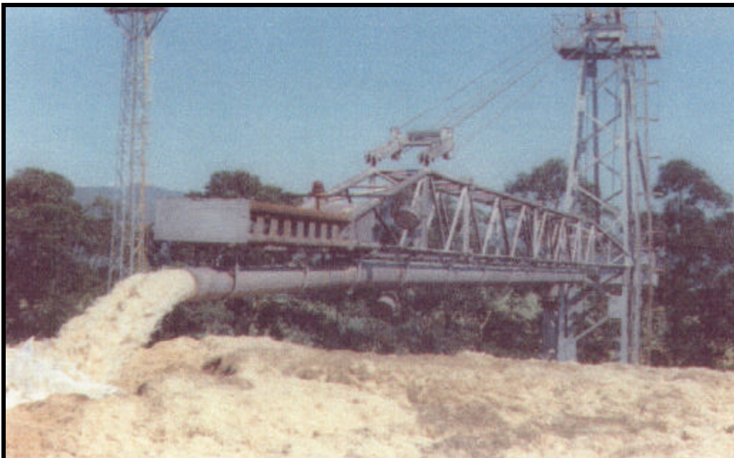
Figure 13 Bagasse Wet Storage
